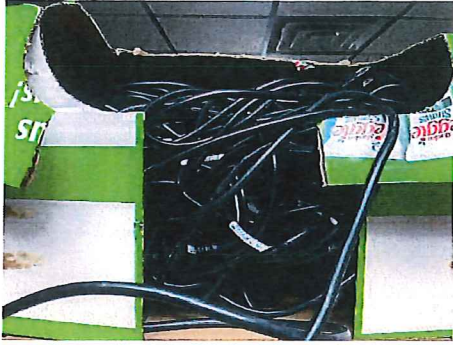
Box of power cables (15)
